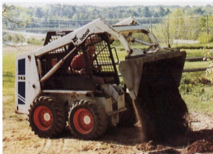
With a borrowed bobcat earth-mover, Dave fills in the now-clean tank site.
