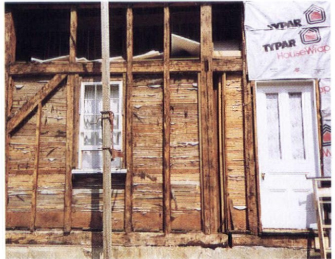
Removing later siding and original sheathing boards exposed the structural frame for inspection and wiring. Note the split-board lath and plaster.
