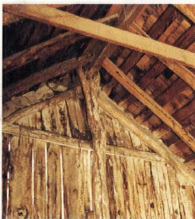
A jacal (top) survives in Los Saenz, Texas, under a new wood shingle roof. A natural fork in the end post supports the ridge pole of a typical 12' by 18' jacal (above).
