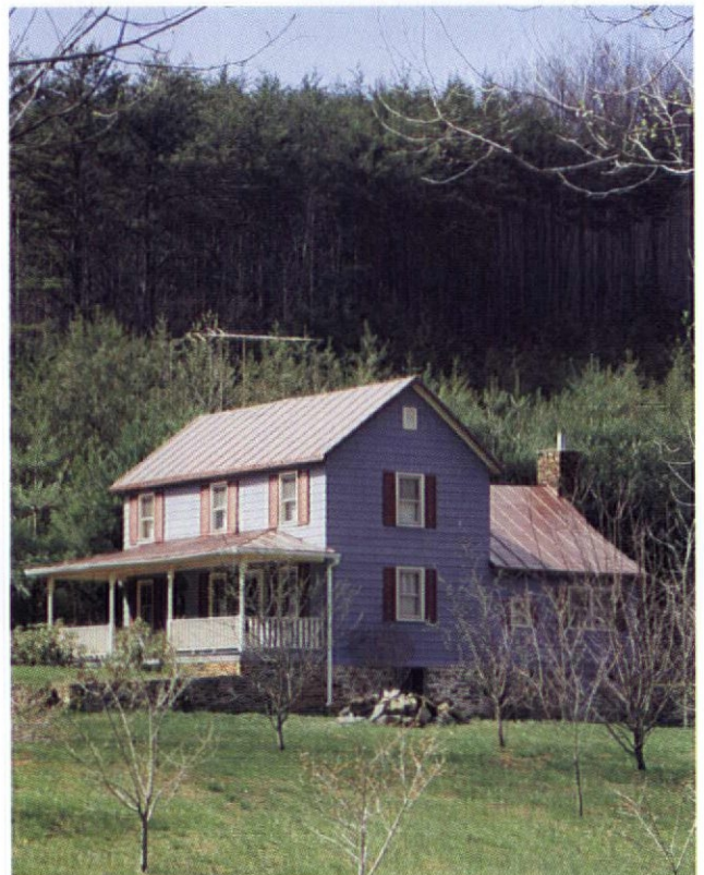
Right: A copper standing seam roof, like this one in Virginia, can last for more than 60 years. Opposite: Tin and galvanized roofs, such as this New Jersey example, need regular painting.
