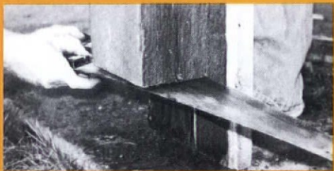
10" rotted bottoms of these load-bearing columns...
