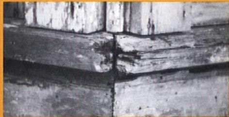
This rotted – and irreplaceable – woodwork...
