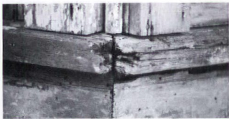
This rotted – and irreplaceable – woodwork...
