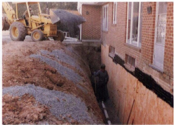
Tuff-N-Dri in place with protection board. Rigid perforated drain pipe is being bedded in gravel.
