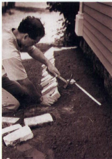
Laying the drip course: contractor Mike Tero digs a furrow and then tamps bricks into place
