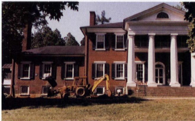
The backhoe begins excavation near the foundation of this Jeffersonian Greek Revival.
