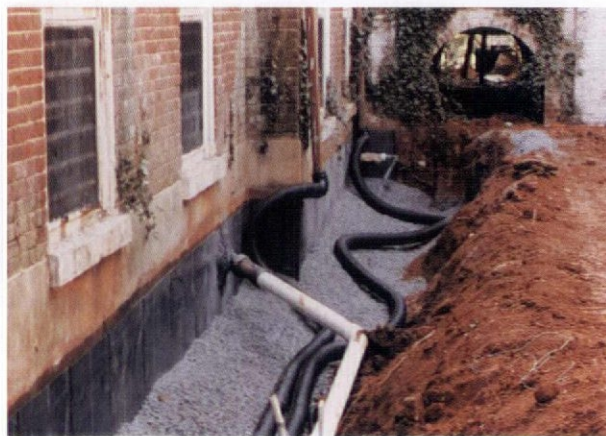
The Bitutbene asphalt/polyethylene membrane in place, with a temporary downspout line visible.
