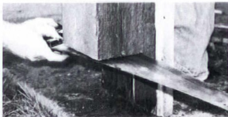
10" rotted bottoms of these load-bearing columns...
