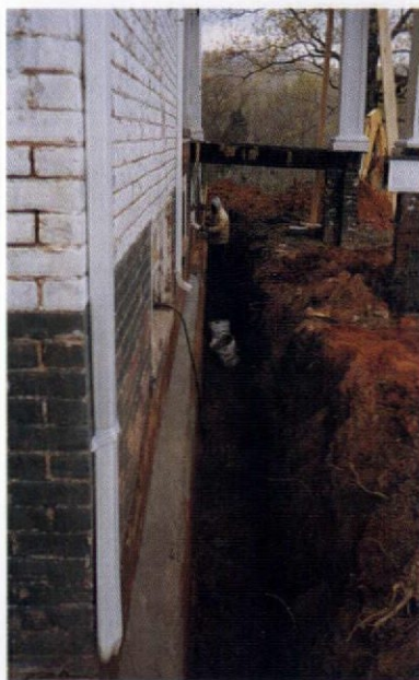
Top, the foundation wall is cleaned with high-pressure water before parging. Middle, note the unevenness of the wall below grade. Above, the brick foundation is parged (plaster-coated).
