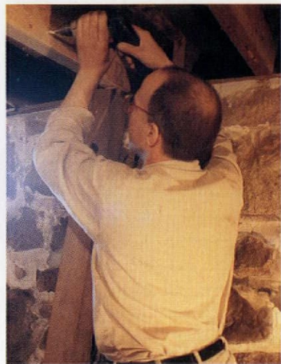
We drilled through the old joist, using the predrilled holes as a template to ensure that the rod holes would line up without the need of a long bit.
