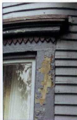
Peeling trim on a tower window, and "chunk" buildup on clapboards.
