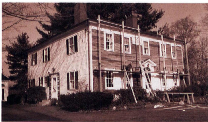
Reclapboarding an Adam house exposed a damaged sill and a whole new project.
