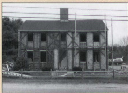
A c. 1815 timber-frame house, sans siding. Note the extensive wind bracing needed for this seacoast site. Photo by John Leeke.
