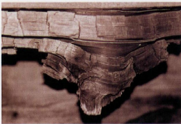
Fungal decay in wood typically produces a chunky, cubic texture. The lower half of this joist has crumbled away, leaving the resin-heavy knot.
