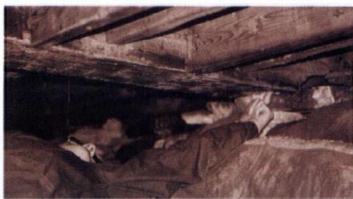
The sill in this damp crawl space has decayed where it joins a girder and is spongy enough to be punctured by a finger.
