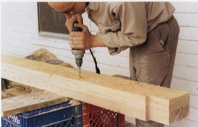
New reinforcement timbers were stacked and predrilled for the threaded rods that would hold them to the inadequate original joist.
