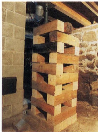
Because we were jacking three floors, we used 20-ton screw jacks and heavy timber cribbing to minimize risk.
