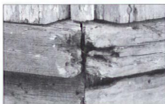
This rotted - and irreplaceable - woodwork...
