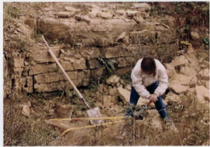
Exploit the natural breaks of horizontal bedding planes by wedging with chisels. A band winch helps when loading stone.
