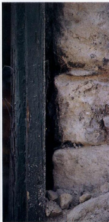
Joints near window and door frames are often large (right) and can be reduced by adding stone or moulding, or pointed as is. Poorly anchored stone (far right) will require backpointing before proceeding further.
