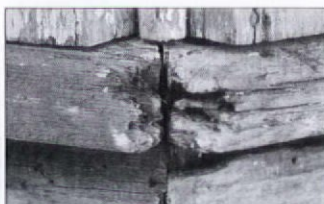
This rotted — and irreplaceable — woodwork...
