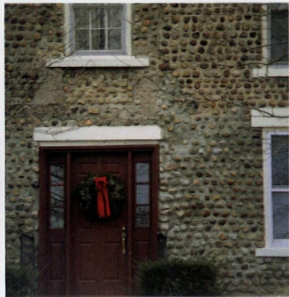
Right: Poorly matching mortar makes a "repair" only worse.
