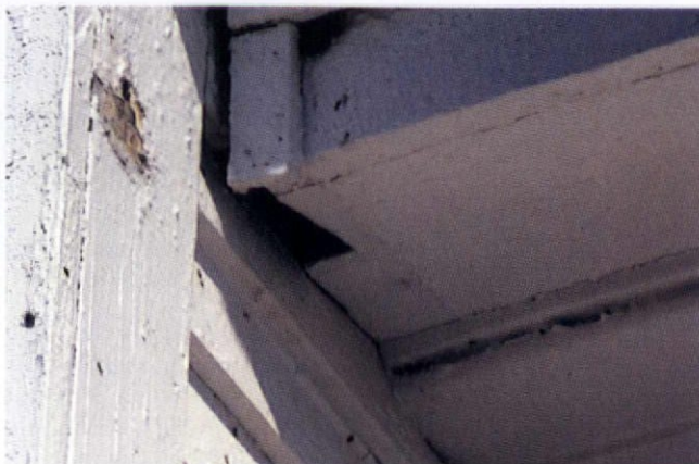
An active bat entrance created by poorly fitting eave soffit trim. Batproofing requires sealing all such gaps.
