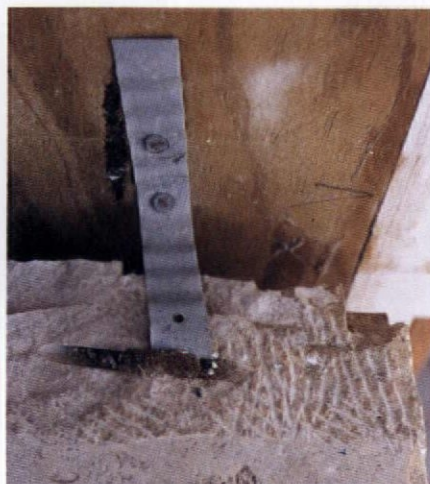
Anchor replacement stone to a frame wall by grinding a pocket into the stone (far left) and securing a brick tie in the cavity with a wedge (left).
