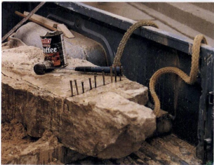
Top: Tools for shaping and setting stone include (left to right): chipping hammer, 2 1/4" set, 2 1/4" tooth chisel, point chisel, 1" tooth chisel, small chipping hammer, pointing trowel. Above: Stone is cut by first scoring both sides, then wedging off waste with cut nails.
