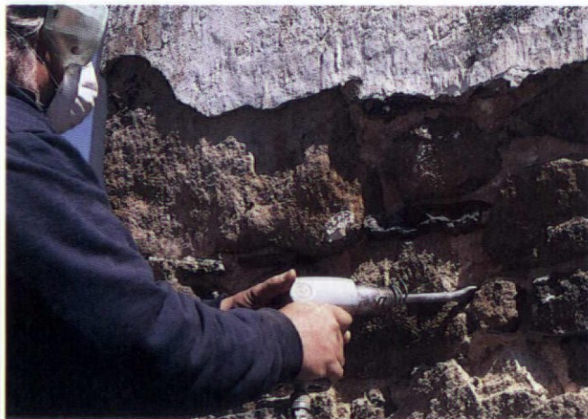
Careful use of a chipping gun removes old mortar, but some hand chiseling is still necessary and does the job best.
