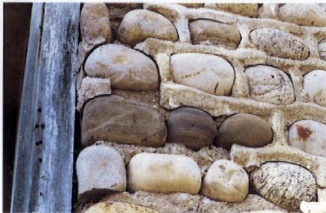
Mortar-joint failure in a cobblestone wall, possibly due to a hardness mismatch between original and repointing mortars.
