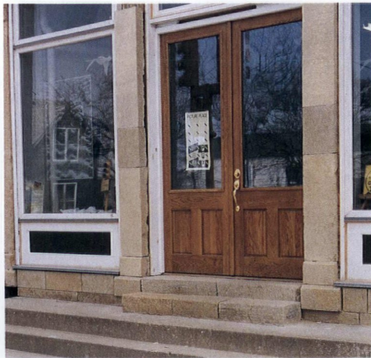
The nearly complete repair showing steps, watercourse, and columns of newly quarried native stone.
