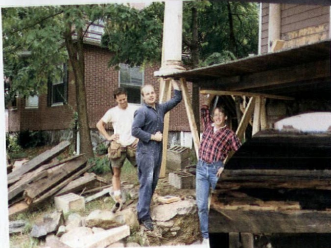
Top: Moss-covered shingles on second-storey gables waiting to be replaced. Above: That's Jack, center, posing with buddies as "better porch support." Inset: This is what we found on the porch when we ripped off the exterior shingles.
