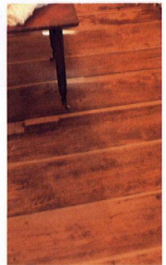
Wood strips were cut into this plank floor because the cracks were a menace to high heels. Widening the cracks to highlight the strips was preferred over attempting a subtle repair.
