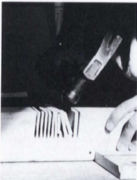
A hammer quickly turns a line of circular saw cuts in framing lumber into a notch.
