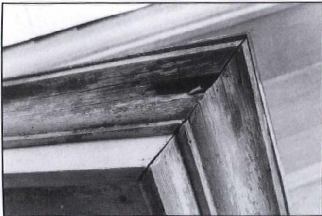
Treatment of this gable-end return cornice moulding will be easier if it's removed.
