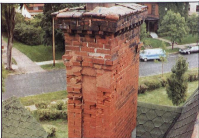
Years of moisture damage and lack of maintenance have devastated this chimney.
