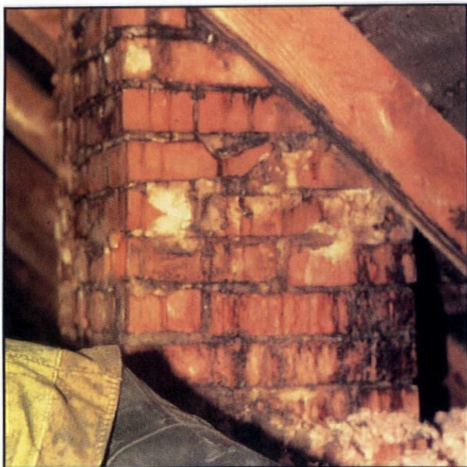
Creosote leaking through mortar joints is a sure sign of problems.
