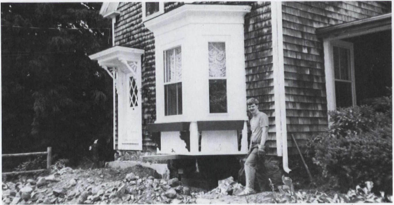
A slight miscalculation during foundation repairs caused this gaping hole, but Chris still manages a smile.
