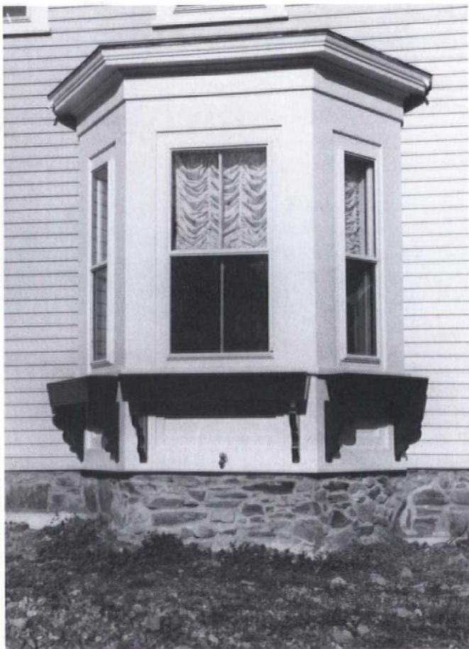
The restored fieldstone foundation and clapboard look as good as new, or should I say old?
