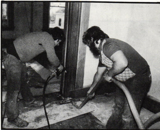
Some contractors pressure rinse after stripping, removing water with a wet vac.
