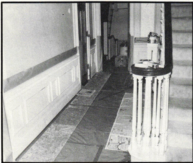
A careful contractor can do extensive paint stripping in a finished house if masking is thorough.
