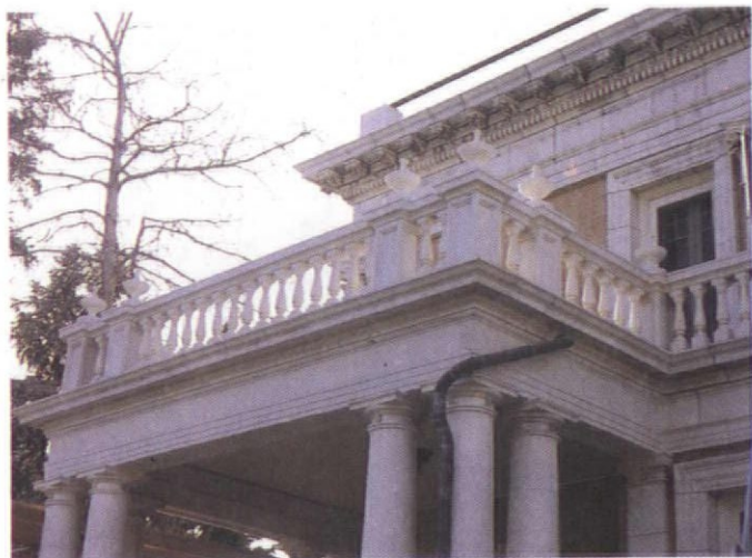
In these photos, we see the new terra-cotta balustrades that adorn the mansion's first- and second-floor porches. The
