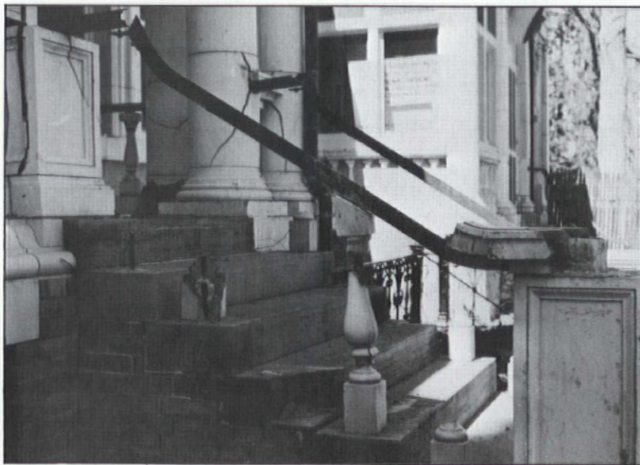
Terra cotta failure: try again, or give up?
