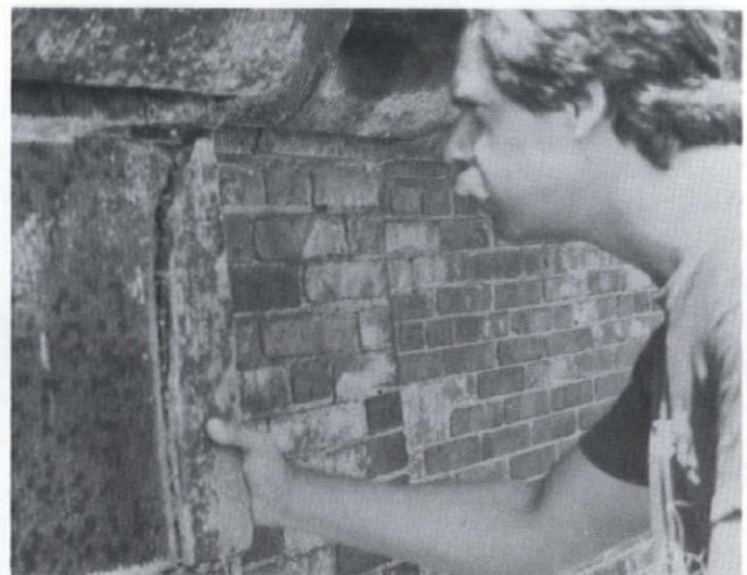
Hands-on inspection of terra cotta. Here, a dangerously-loose piece is discovered.
