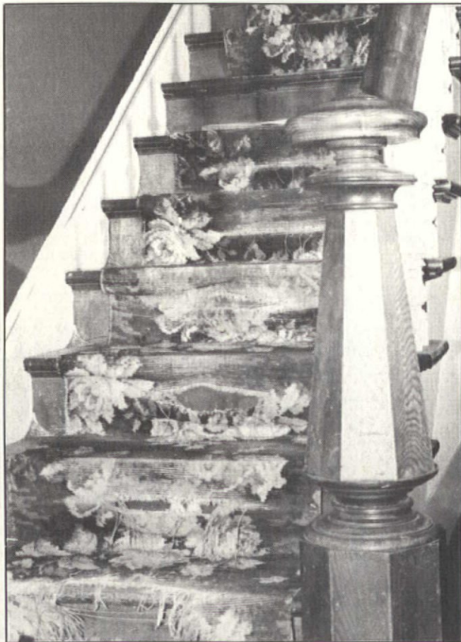
The worn carpet on the stairs is a last remnant of the house's original carpet. Note the brass dust corners, designed to make sweeping easier.
