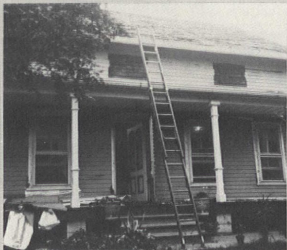
Trim has since been restored to the blind eyebrow windows.
