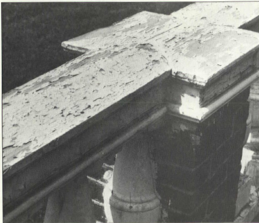
Weathering is worst on exposed horizontal surfaces. This rail must be scraped, treated with a water repellent, and primed before painting.
