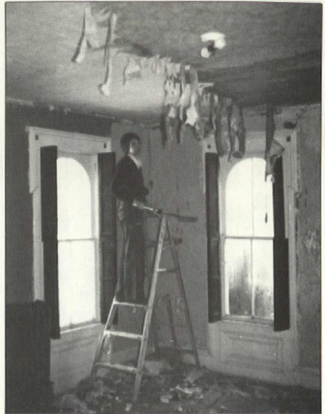
Brenda Ferre used a paint roller dipped in hot water to loosen wallpaper from the ceiling. Messy, but looks like it works!
