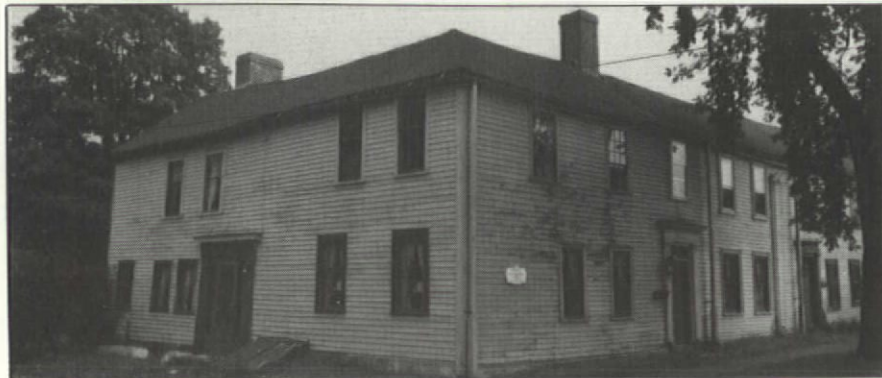
Paint applied over obvious problems will fail again -- unless inspection reveals the cause to be corrected first.
