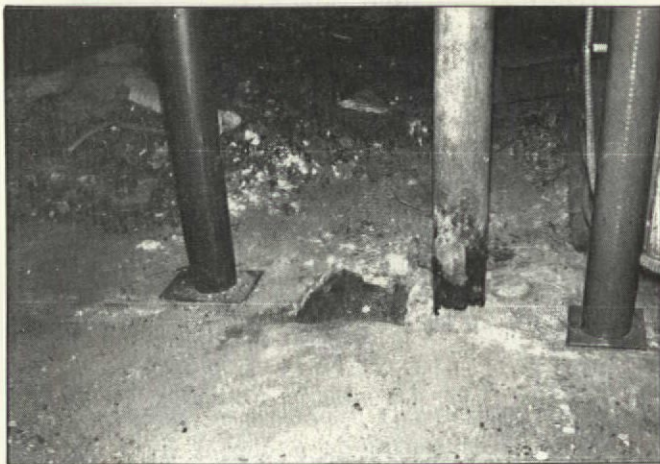
With a rusted foundation post like this one (center, surrounded by new jack posts), it's no wonder the living room sank two inches.
