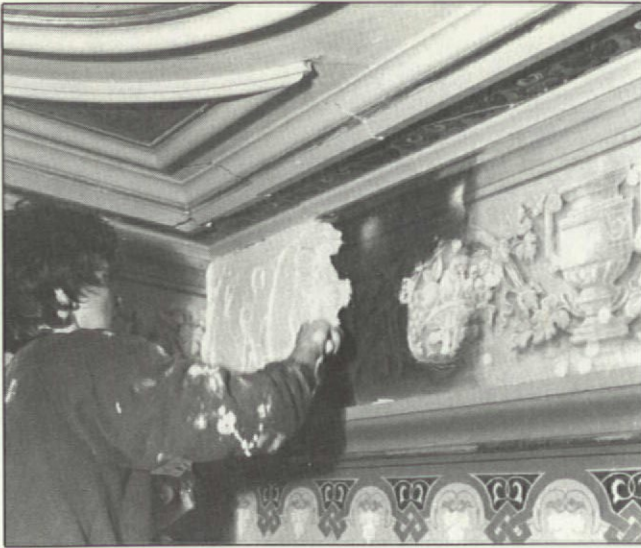
A plaster poultice is used to rescue the trompe l'oeil frieze border in one room of Connecticut's Lockwood-Matthews Mansion (Richard Bergmann, Restoration Architect). Louise Stoltz is applying the poultice. (Note the already-cleaned section of border to her right.)
