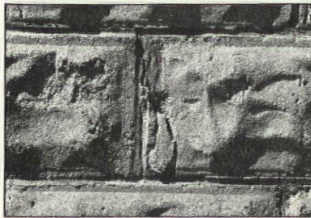
A broken corner in a rock-faced block that's a good candidate for simple patching.
