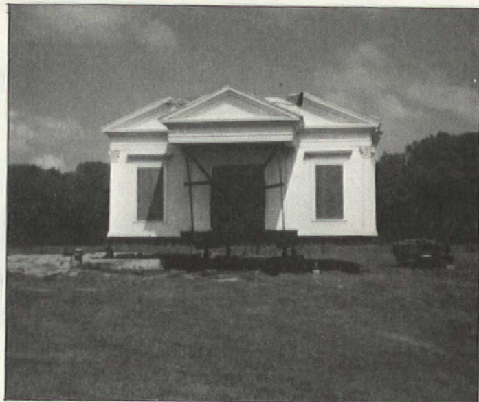
Left: The house is on the road to the O'Neles' land on the outskirts of town. Above: The house spent its first night after the move on four hydraulic jacks.
