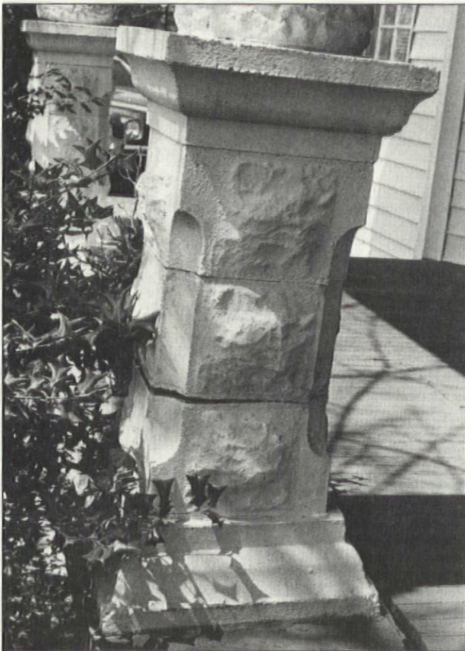
A failing porch foundation caused the blocks in this post to separate. The foundation should be fixed before the post blocks are reset.
