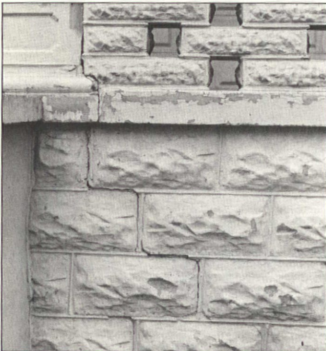
Settlement commonly causes joints to open, and deterioration starts if cracks are not filled to keep water out.
