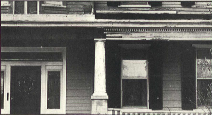
But up close, the problems really stood out: Paint that was dingy, mildewed, and peeling, and wood that was rotted or missing altogether.
