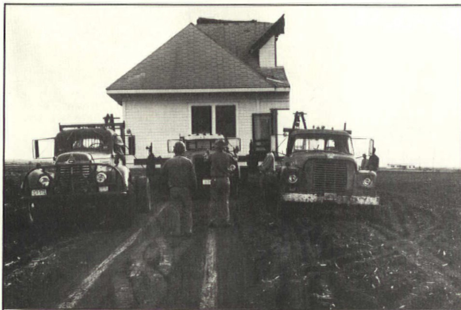
Half the house is stuck in the mud. It took more than these two trucks to budge it.
