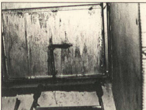
The downward-opening hatch cover described earlier. Details of its manufacture are a trade secret. Top, note the flat, un-pry-able metal cover faced by the would-be thief. Lower photo was taken from inside closet that leads to roof hatch. Thanks to Dr. Arthur Hazlewood, New York.
