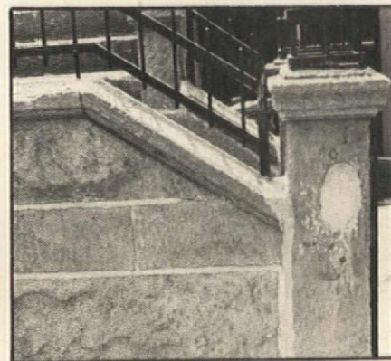
These portland cement patches had been made by a previous owner before the steps were painted. Sandblasting exposed them, to the present owner's dismayed surprise.
