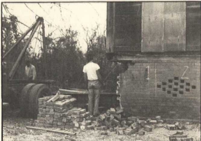
This photo of the disassembly of the brick foundation also shows one of the steel beams which will support the raised house. (Note the numbering of different sections of the foundation.)
