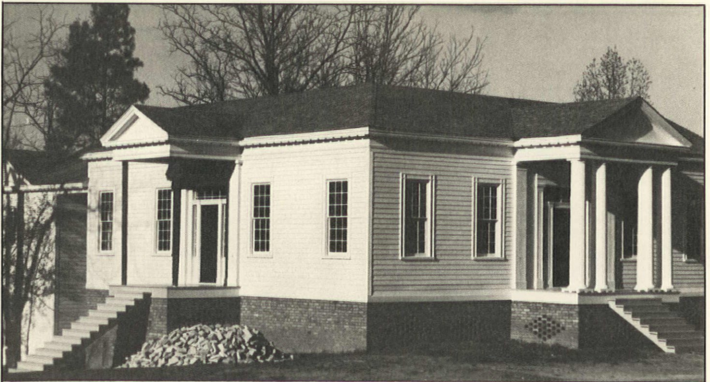
This photo shows the relocated Griess house when work was in progress. The
