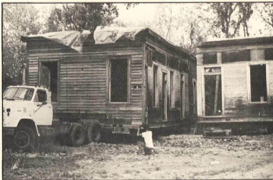
A section of the Griess' house starts on its way to Eutaw.
