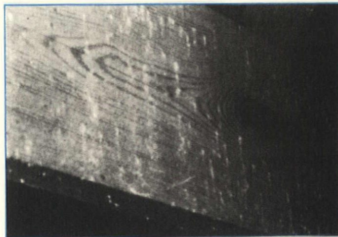
Finely powdered wood dust streaming from exit holes is the hallmark of the Anobiid beetle—also referred to as the "Powderpost beetle." The greater the number of exit holes, the greater the age of the infestation—and the greater the damage is likely to be.
