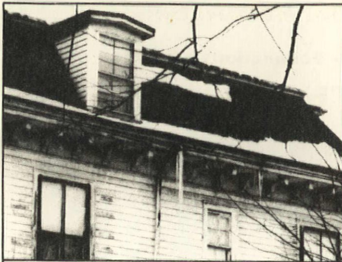
Icicles provide dramatic evidence that water is leaking into the cornice of this old house. Gutter repair or re-building, as well as cornice repair, will be required.
