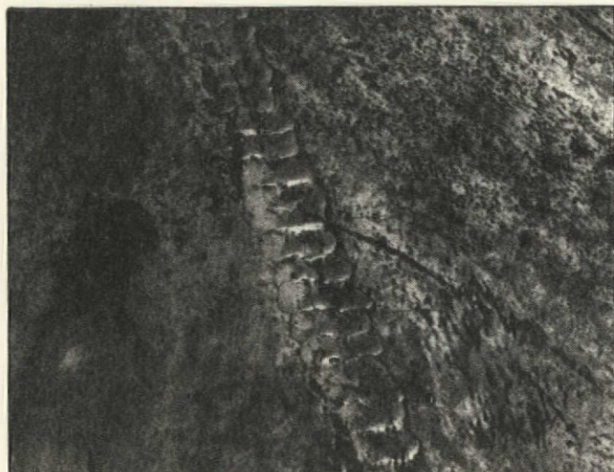
19TH CENTURY soldered joints were nearly invisible; this is a modern repair. Wide joints increase likelihood of galvanic action and failure due to differential expansion of solder and terneplate.
