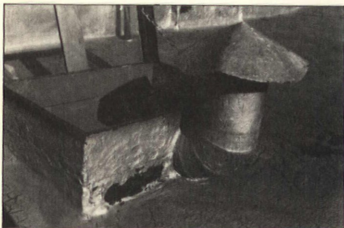
THE TINPLATE FLASHING of the roof hatch has been corroded away (in front of the vent) by the action of an asphalt coating and water.
