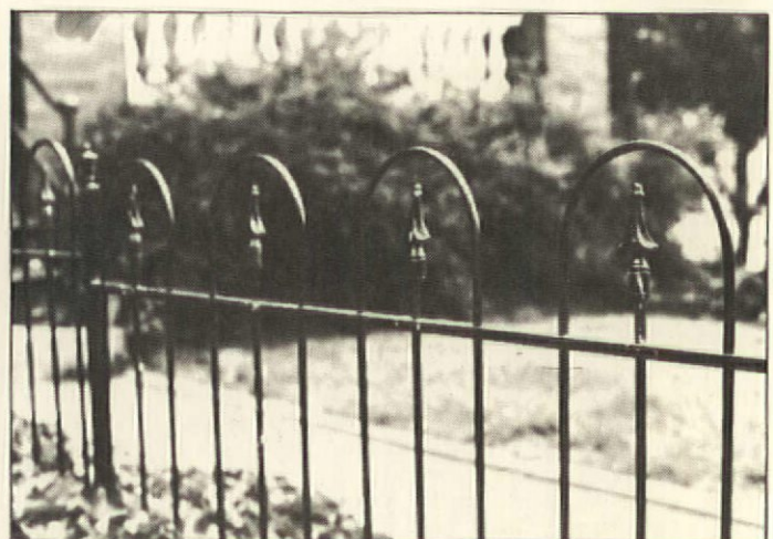
A simple hairpin-and-spike fence, suspended from square posts like those used for modern iron rails
