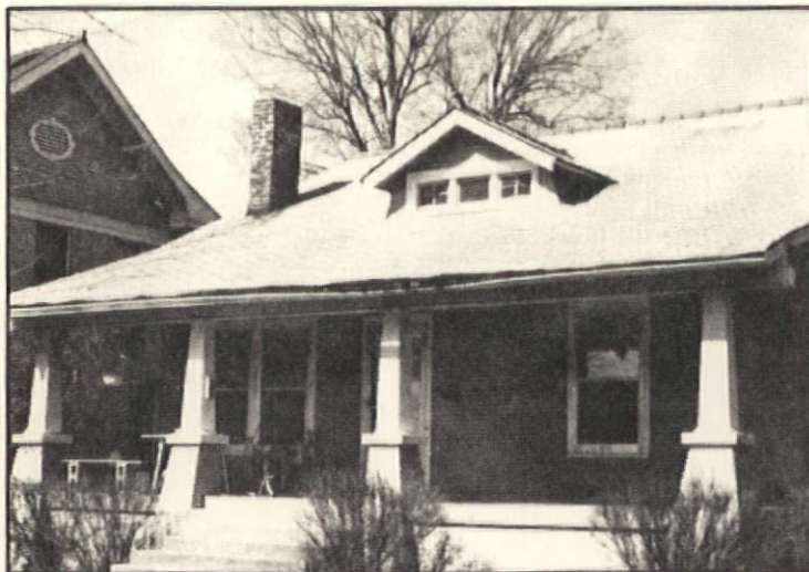
Roofs frequently fail at the eaves first. This bungalow has a sagging gutter that collects water in the center. Bumpy look at the eave indicates a new roof has been applied over a deteriorated old roof--which is still rotting.
