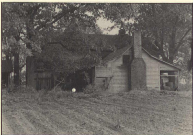
The rundown addition containing the bathroom and kitchen were removed from the original part of the house.
