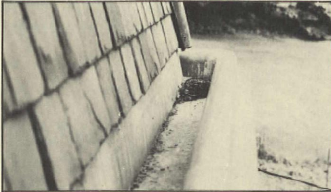
This built-in gutter at the base of a slate Mansard roof is lined with lead-coated copper for maximum durability.
