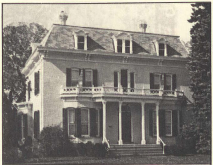
The Loop-Harrison house (1872) in Port Sanilac, Mich., has built-in gutters in the cornice at the base of the handsome Mansard roof. While giving a clean uncluttered look to the front of the house, such gutters often leak water into the structure.
