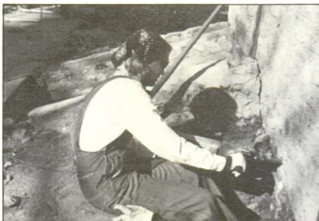
Norma did much of the preliminary work before professionals came on the job. Here she is drilling holes for the power lines through 18-20 in. of the fieldstone. It was a three hour job.
