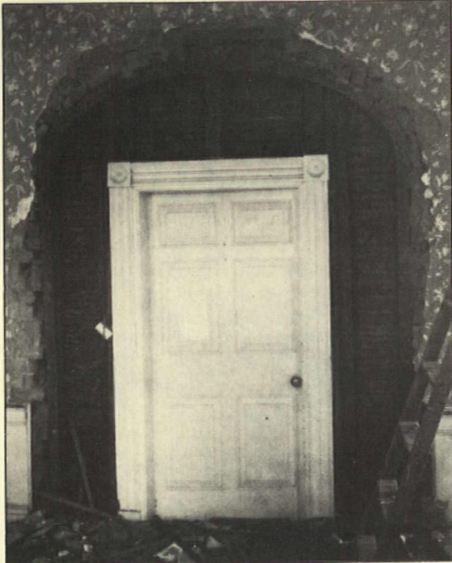
The wood trim on the arch had been hacked away but, after the door was removed and the wall knocked away, the panelled opening turned out to have its original framing intact.
