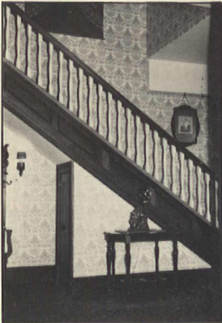
15-ft. panel under stair balusters came off in one piece for stripping after trim pieces were removed.
