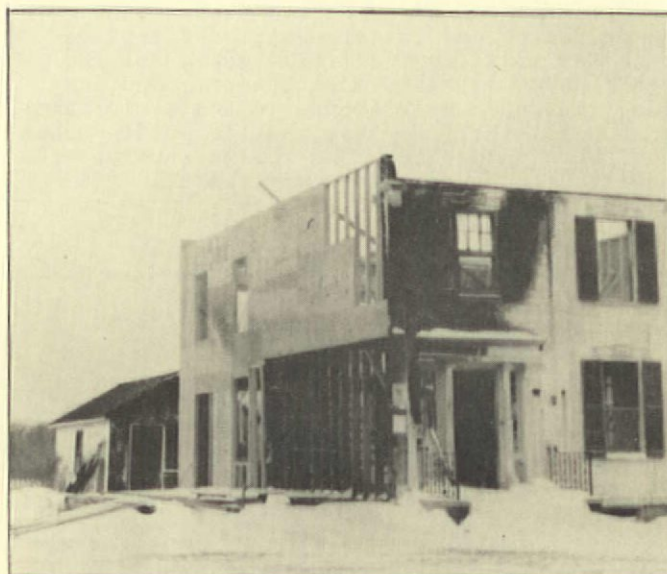
The house now shows the rebuilt portion, with the pediment removed for copying and salvage. The heavy bracing and studding is original.
