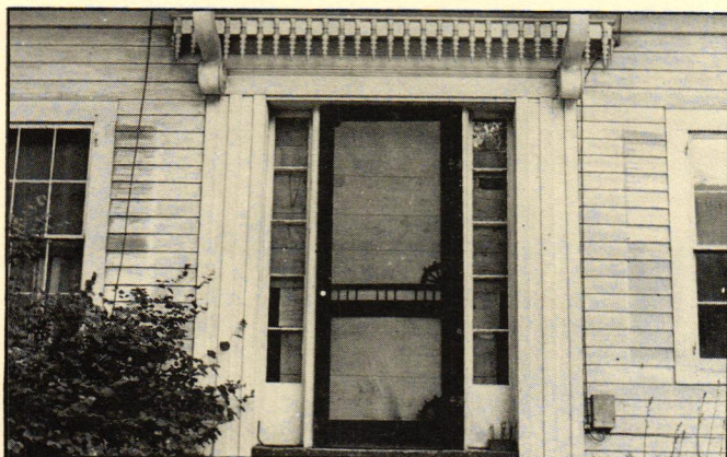
Built in the early 1800's, house was a derelict when purchased: Shutters and front door had been ripped off. Amazingly, the turned icicle trim—part of Swiss Chalet theme—had survived intact.
