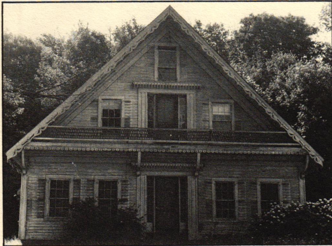
The Chalet, on its original site, showing the symptoms of an abandoned house: Broken windows, boarded doors and peeling paint.
