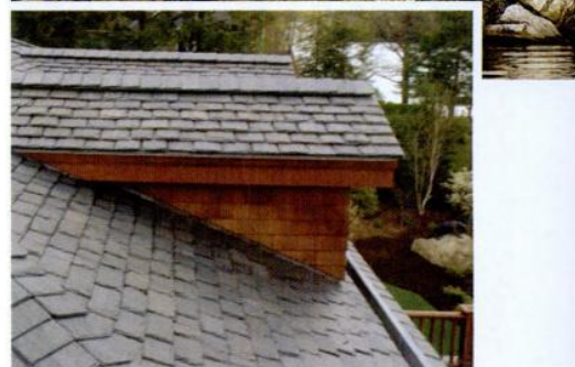
TOP: A pre-painted terne roof in one of 20 colors available from Follansbee.
