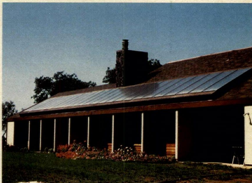
Flat-plate collectors , shown installed, are part of a heating/cooling system which also heats domestic hot water and a swimming pool. System is controlled by a computerized HELIO-PAK module. Heliodyne. Circle 239 on reader service card
