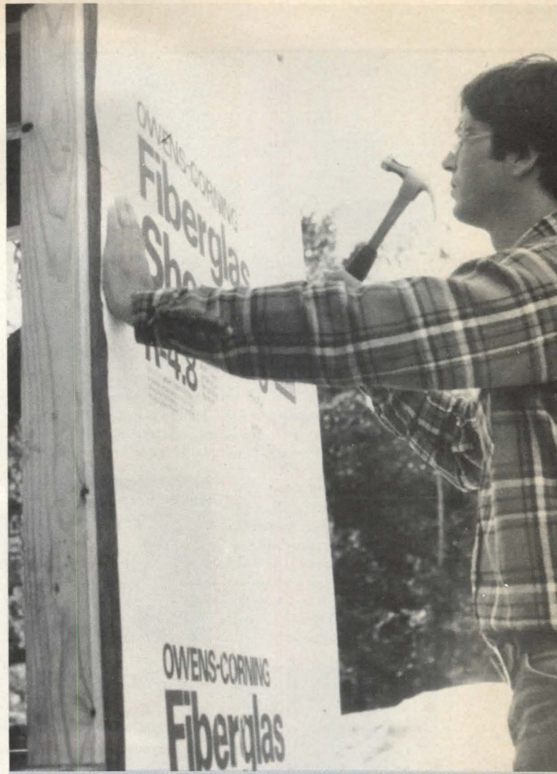
Nailing: Sheathing is applied to studs with 1 1/4" galvanized roofing nails that have 3/8" heads.
