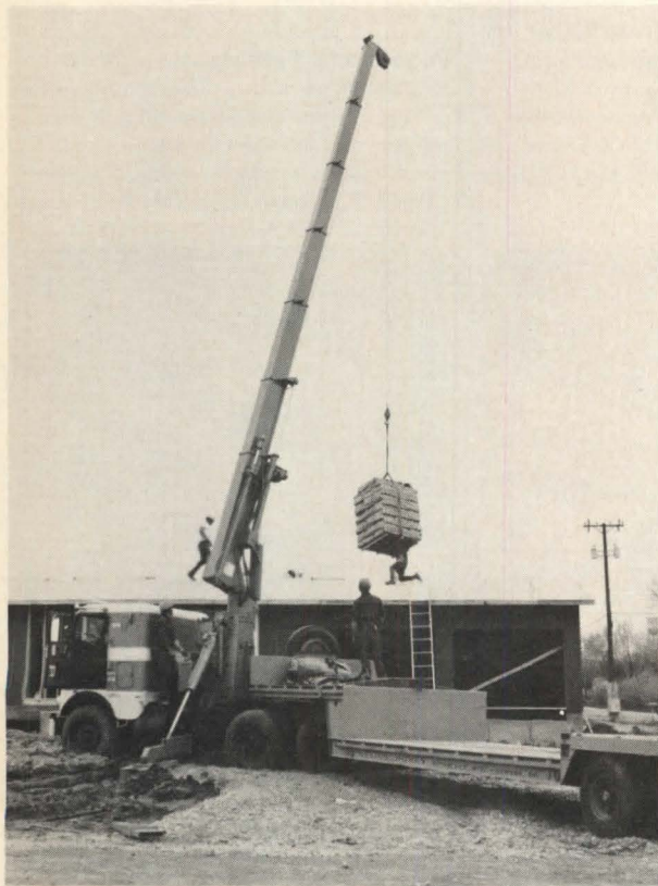
Tractor-mounted crane, "Model 7-11" (above), is specially designed to speed the erection of panelized homes. Machine can hold up to 11 tons at 70°, and 2,000 lbs. at a 42' radius. Retractable crane stores over cab. Paxton-Mitchell. Circle 272 on reader service card
