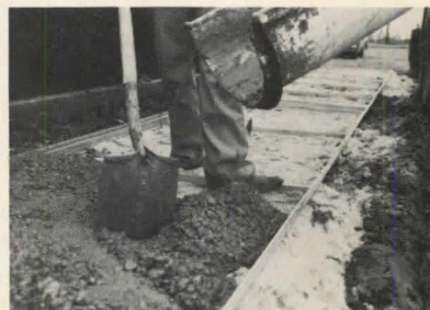
Concrete forming system (above) is designed to remain in place as part of the finished sidewalk. Leav-er-rite. Circle 236 on reader service card
