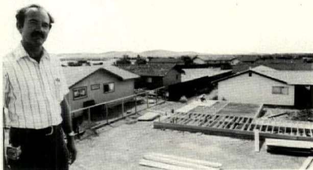
Jerry Brown, construction manager for the D.L. Nelson Corp., at the jobsite in Suisun, Calif. Insulated Plen-Wood system is under construction at right.
