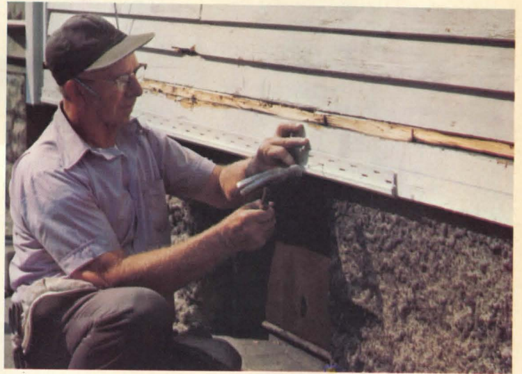
3. Position starter strip with top edge on the chalk line. Do not nail too tight; stop when hammer head touches edges of nailing strips.
