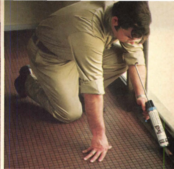
seal around tilework,
