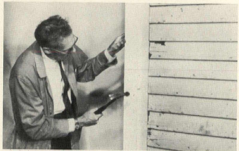
2. Corner posts. Place posts on all inside and outside corners, allowing \frac{1}{4} " at the top. Position the post by placing nail at top of upper slot, placing all other nails in the center of the slots.
