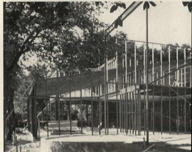
1. Marbridge Foundation Dormitory, Austin, Tex. Architect: Barnes, Landes, Goodman, Youngblood, A.I.A., Austin, Tex. Contractor: Star-Field Constructors, Austin, Tex.
