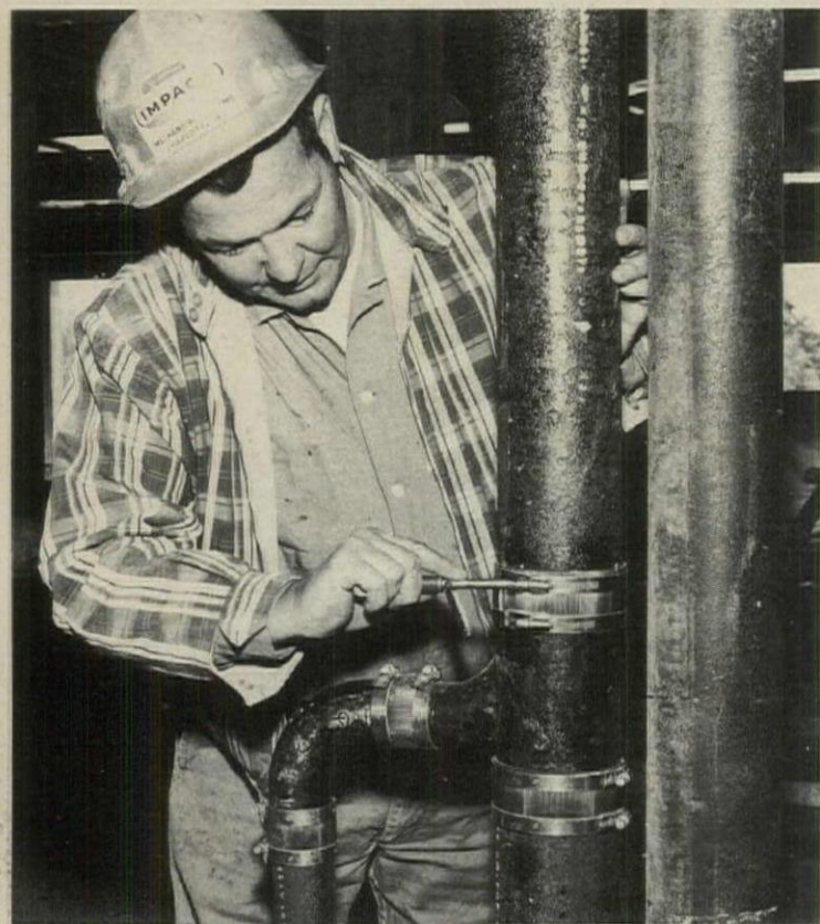
Torque wrench is used to tighten band clamps around coupling. System is fast—plumbers can job-assemble trees rather than prefab them in shop.
