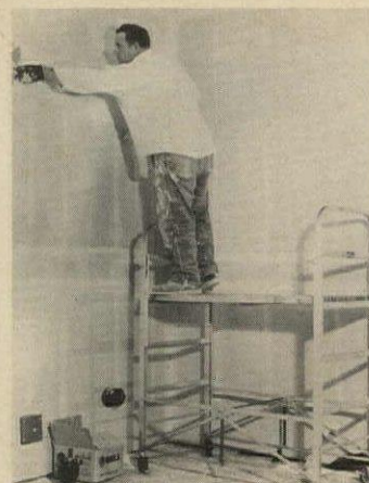
Portable platform is a combination scaffold, ladder and hand truck, lets workmen reach up to 12'. Made of aluminum, it will hold 1,000 lbs., has lockable casters, will fold up compactly, weighs only 60 lbs. American Mfg., Tacoma, Wash. Circle 235 on Reader Service card
