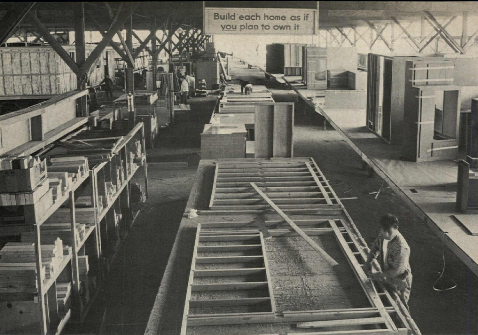
12-STATION ASSEMBLY LINE (plan, below) for Long's mobile homes is in a 30,000-sq.-ft. plant formerly used for prefabricating conventional houses.
