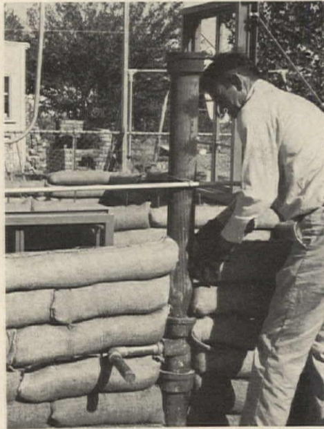
5. PLUMBING and wiring conduits are pressed into place between sacks as walls progress.
