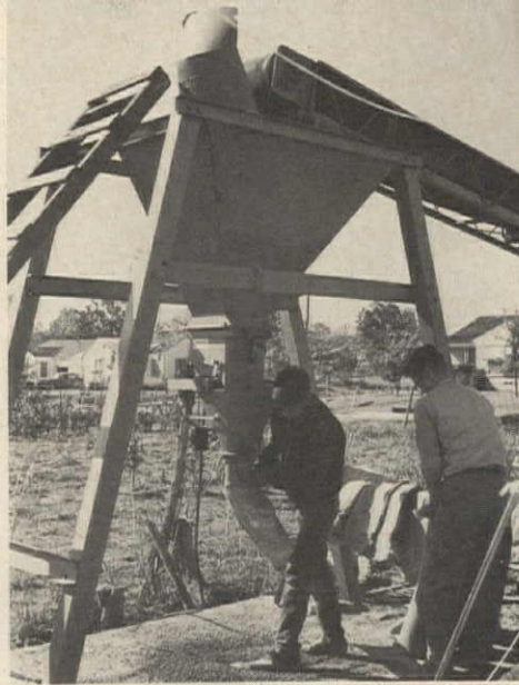
2. BURLAP SACKS —24" long, 6" in diameter—are filled on site. They weigh about 50 lbs.
