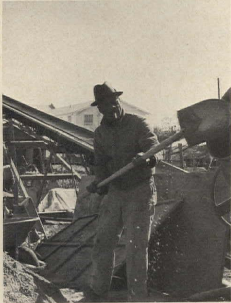
1. DRY CONCRETE MIX with 3,000 psi rating is fed into a hopper by elevated conveyor.
