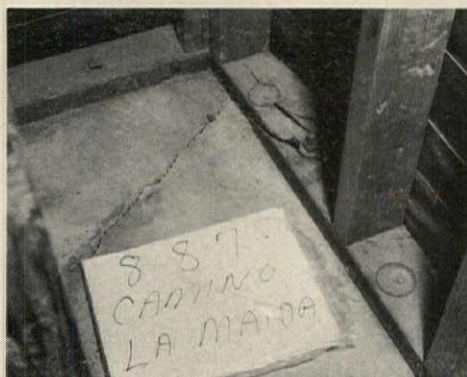
CRACKED SLAB and other serious structural defects led homeowners to sue Great Western S&L, which financed a 250-unit project in California.
