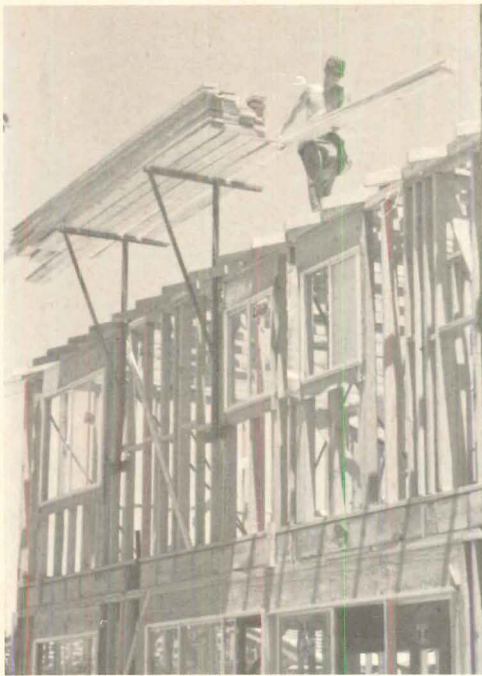
ROOF-LEVEL MATERIALS RACK
