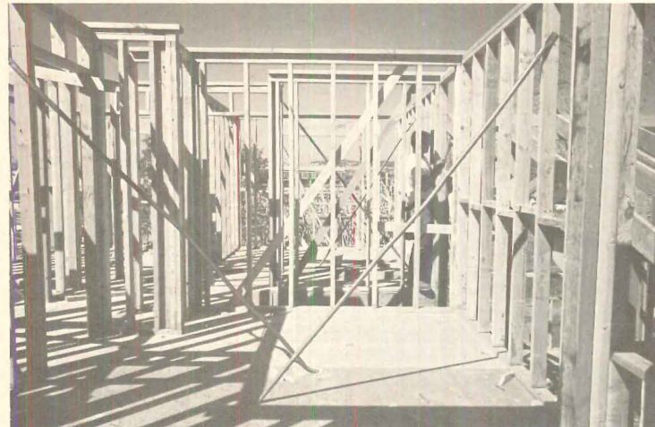
CONDUIT TURNED INTO SHORING
