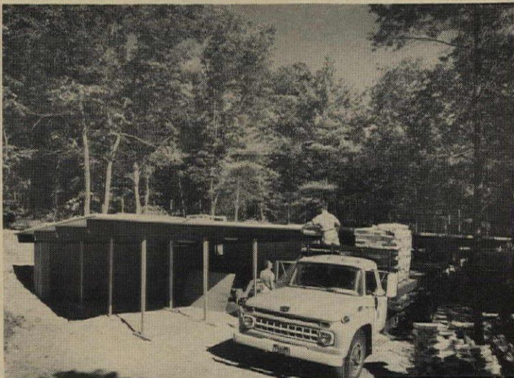
PRECUT ROOF BEAMS are set up on post-and-beam ridge. Wall panels are built in the shop so that quality of window millwork can be maintained.
