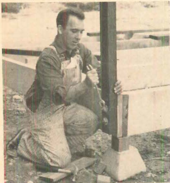
Framing post is joined to double 2x12 sill with two 9"-long bolts.
