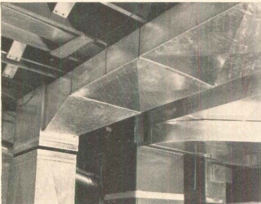
All the ductwork throughout this home—for both heating and cooling—is made from Reynolds Aluminum.
