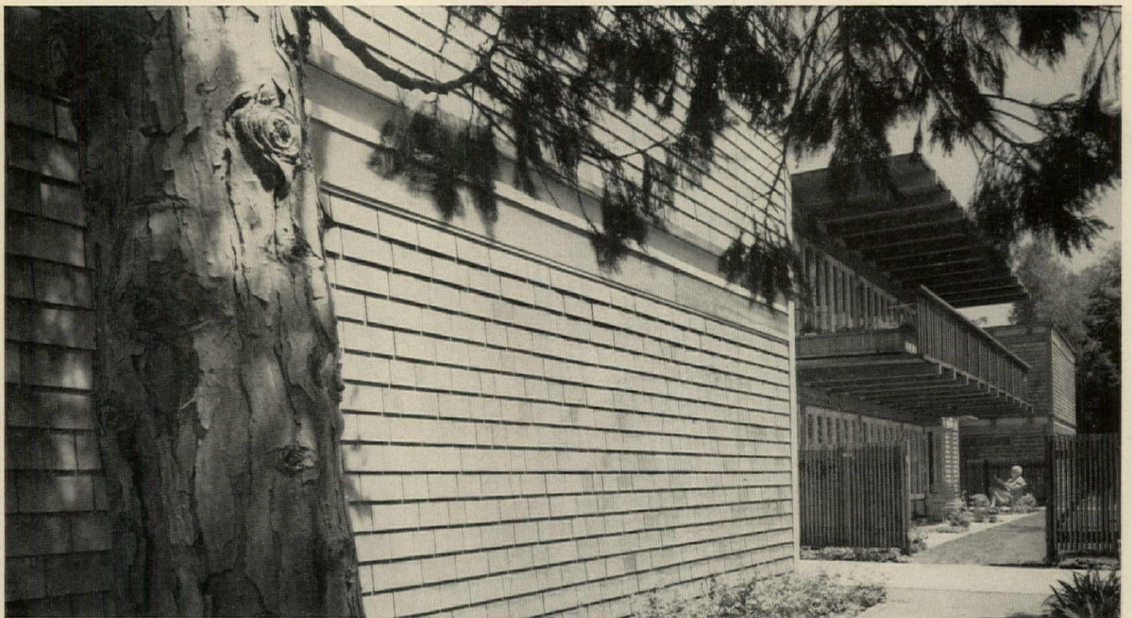
Single-coursed sidewall, Retirement Apartment, Menlo Park, California / Architect: Skidmore, Owings & Merrill / Contractor: Barrett Construction Company
