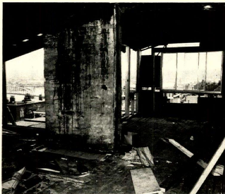
BEFORE , the living room was an attic. Balcony was built on beefed-up roof of second floor; walls were opened up and chimney opened for new fireplace.
