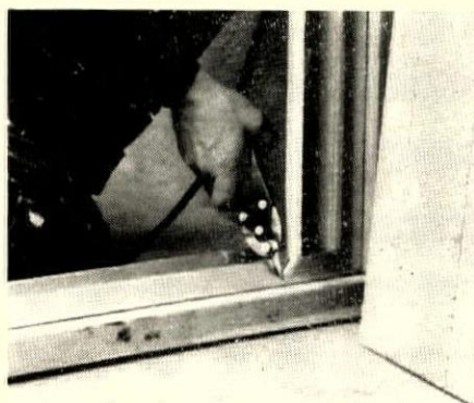
3. STEEL CHANNELS are cut to form tabs which are bent in to hold studs in place.
