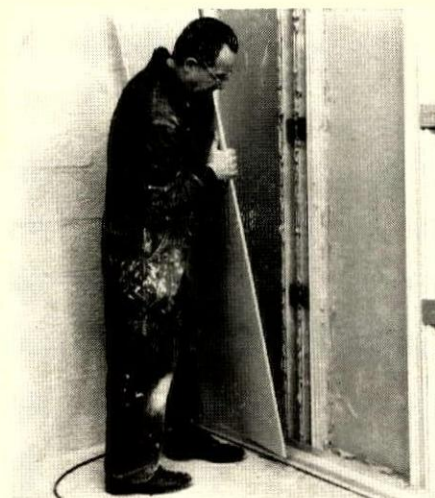
5. ADHESIVE is applied to edges of studs and gypsum skin is put in place.
