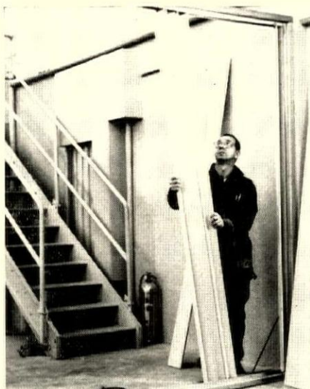
2. STUDS slide into steel channels screwed to floor and ceiling. Studs are 24" oc.
