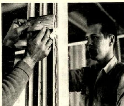
4. STEEL SCREW-PLATES are mounted on both sides of studs at 2', 4', and 6' levels.
