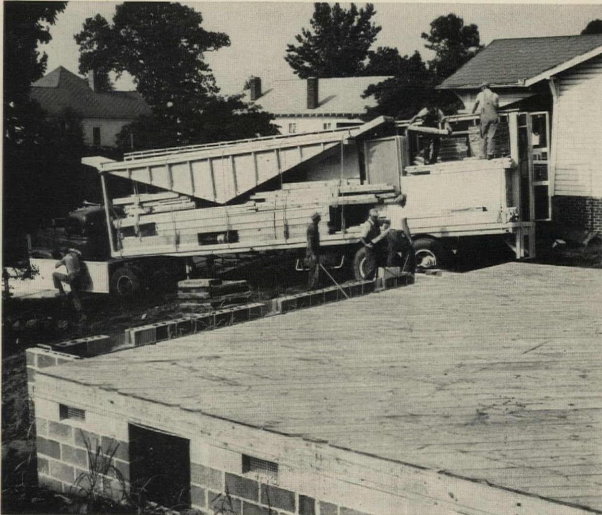
MANUFACTURED HOMES help solve the problem of scheduling and delivery to scattered lots: everything is on one truck.
