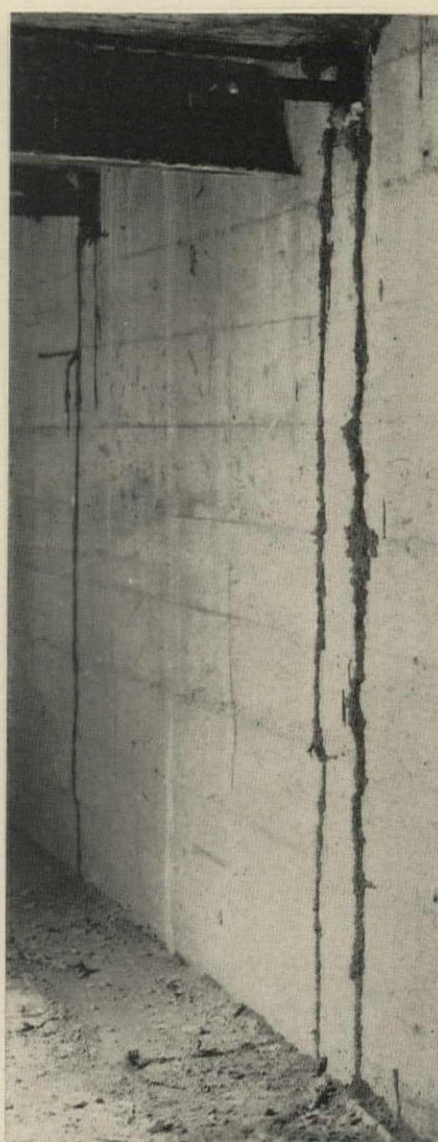
TERMITE TUBES bridge gap between wood in house and moisture supply in the earth.
