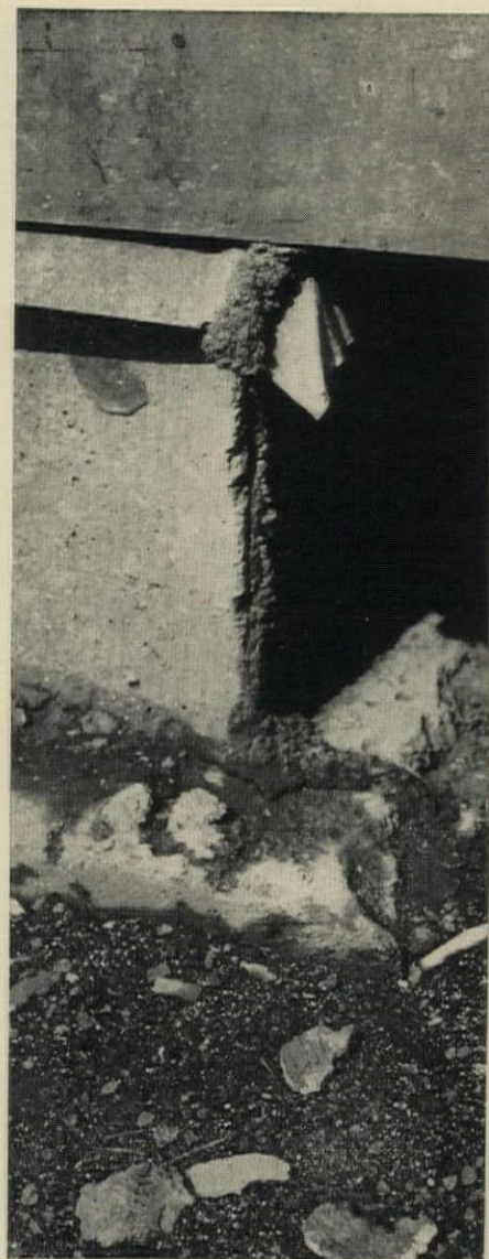
SHIELDS BENT OR DAMAGED by later construction make termite entry easy.
