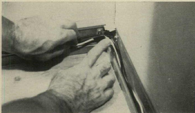
3. COLOR-CODED WIRES are then dropped in base channels. The wires are uncut. Fiber insulators protect wires at channel corners.
