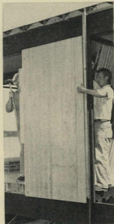
WALL PANELS fit between roof and floor girders (drawings above and below).
