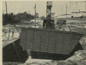
... the treatment plant is quickly installed.
