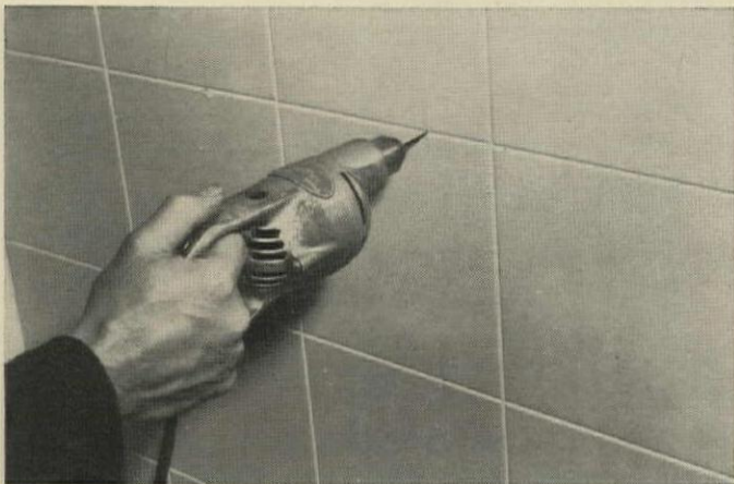
HOLES ARE DRILLED in grout line for plated nails if wall is not true.
