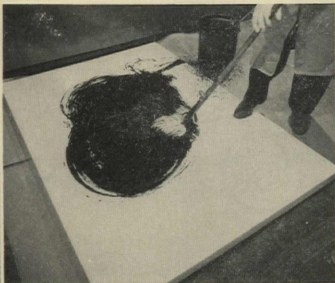
DIRECT HOT MOPPING for built-up roofing is possible with new Thurane. Rigid board will carry weight of wheelbarrow without indenting.
