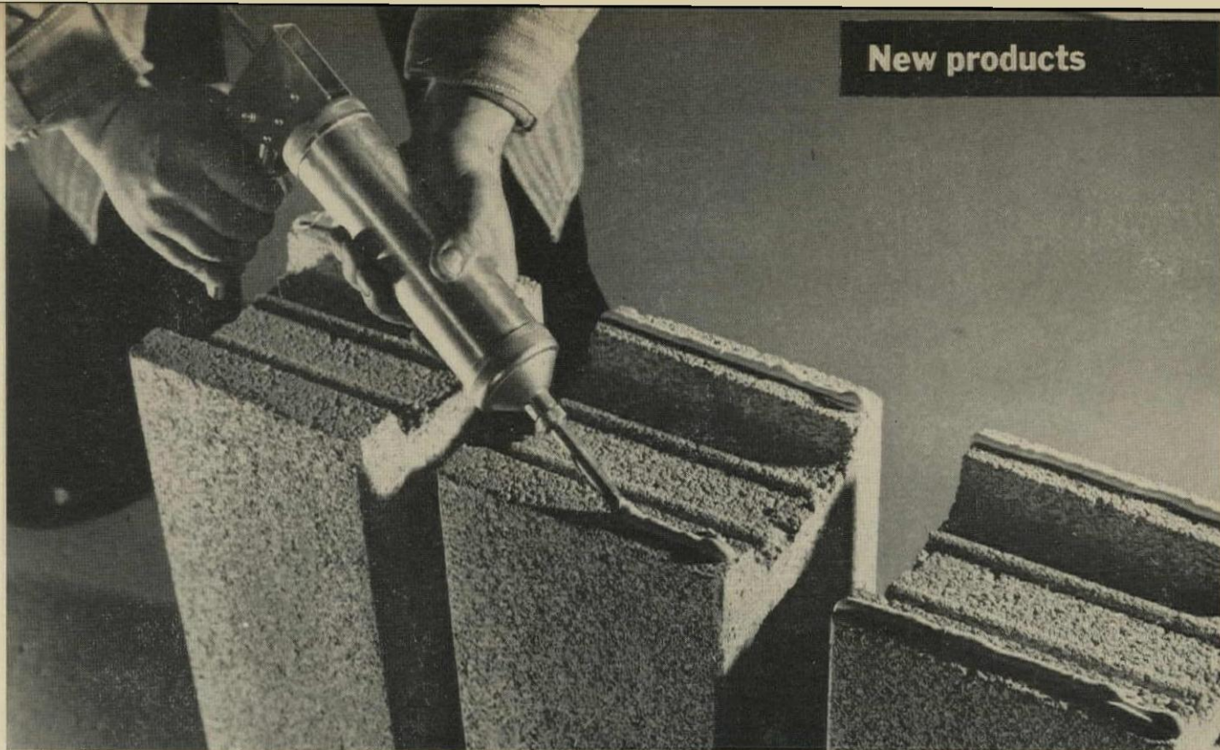
CAULKING GUN serves to spread a thin line of plastic mortar on the block. Pot life allows ample time; the mortar sets in 24 hours.
