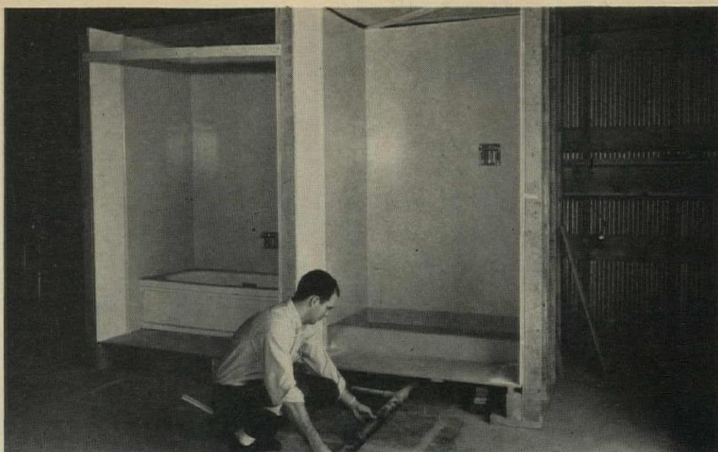
1 EPOXY GLOSS PAINT applied to drywall is watertight, but shows flaws in drywall taping.
