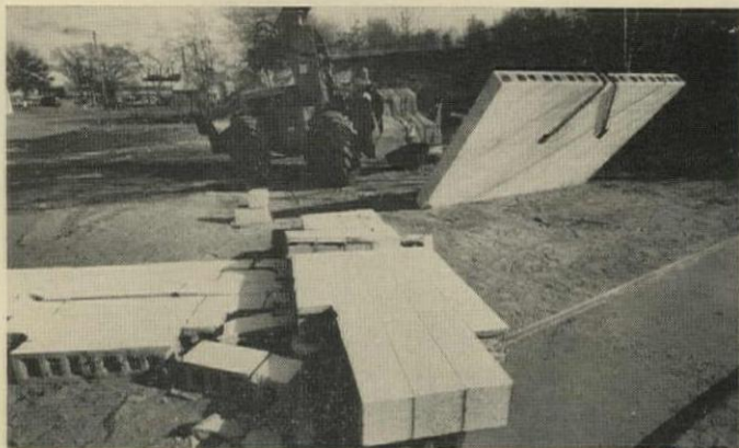
HIGH STRENGTH is shown by tilted wall. Plastic bond resists shear load where conventional mortar, foreground, has failed at the joints.
