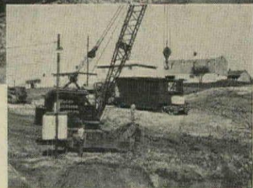
Delivered to the installation site on time.
