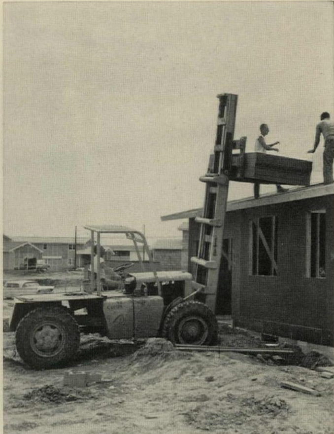
JOB-SPOT DELIVERY by big wheeled lift gives workmen a full roof of sheathing in a single pass. Unit can carry 3-tons over rough terrain.
