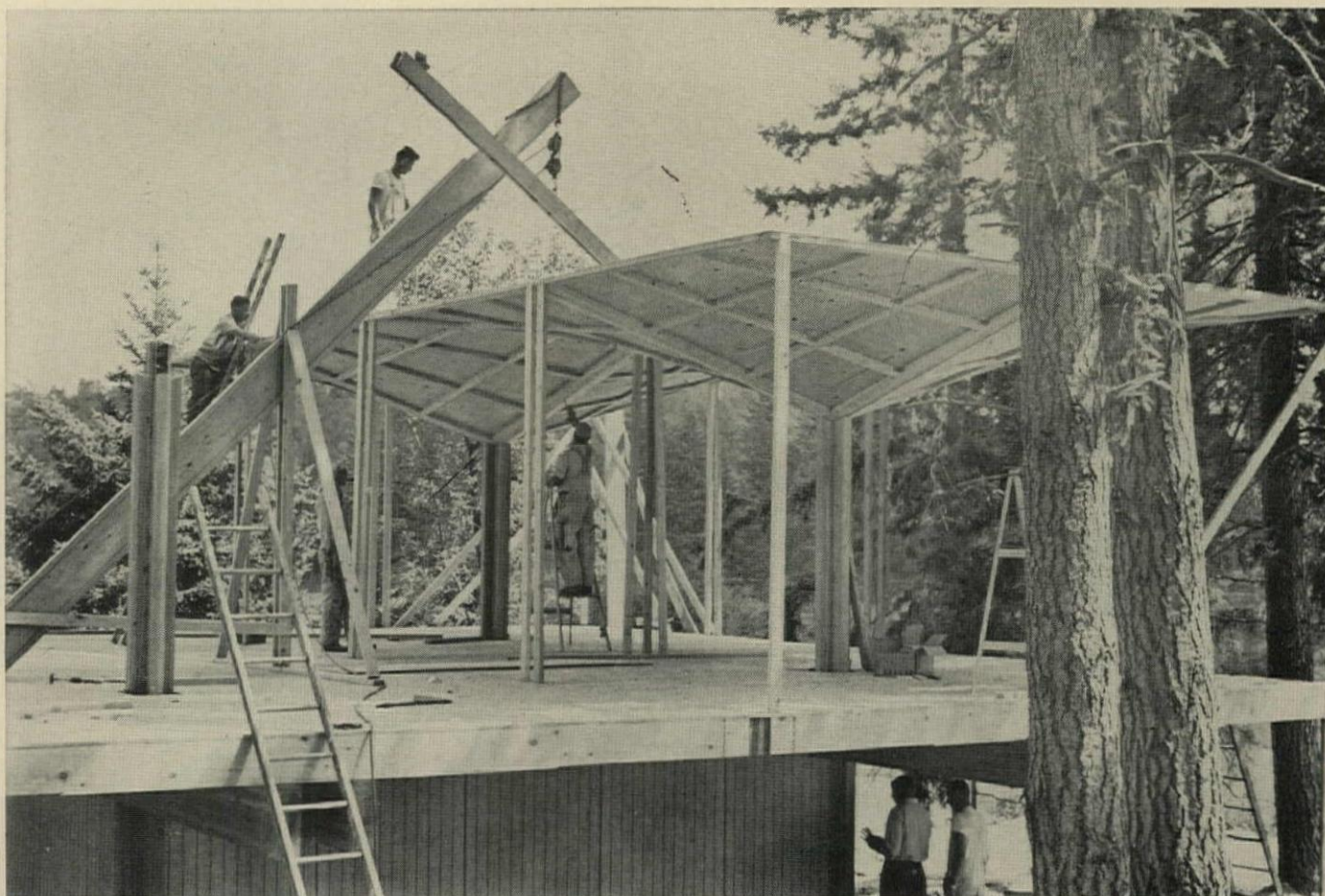
HYPERBOLIC-PARABOLOID ROOF needs no bearing walls, supports roof load on four posts. 2x4 shoring positions two of four h-ps.
