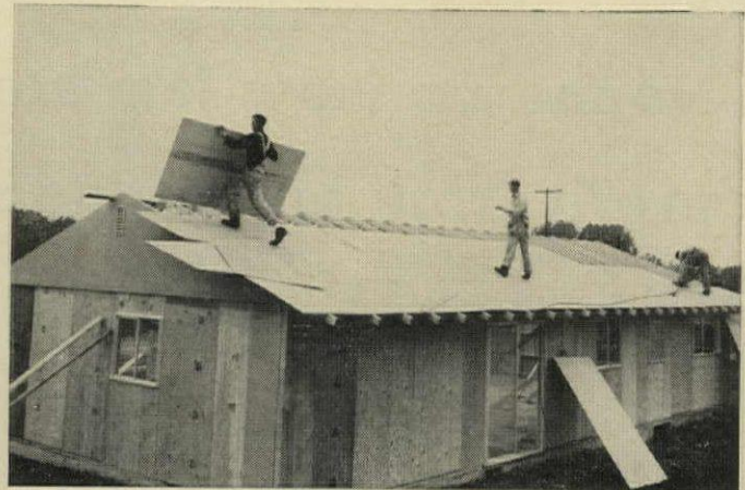
ROOF SHEATHING , stacked against house so crew can reach it easily, is quickly placed and fastened with power nailers.
