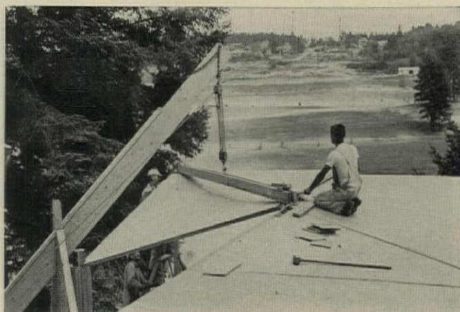
EXPERIMENTAL BOOM lifts roof panels into place. Four 10'x10' panels form each h-p roof section. Sheet metal splice strips will cover joints.
