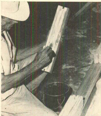
BLOCKS ARE GLUED with a waterproof adhesive that assures a rigid finished wall. Glue is applied to block edges, not tongue.
