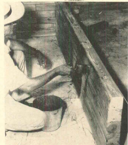
WALL IS FINISHED with wood preservative and water repellent to make it resistant to termites and rot, more stable dimensionally.
