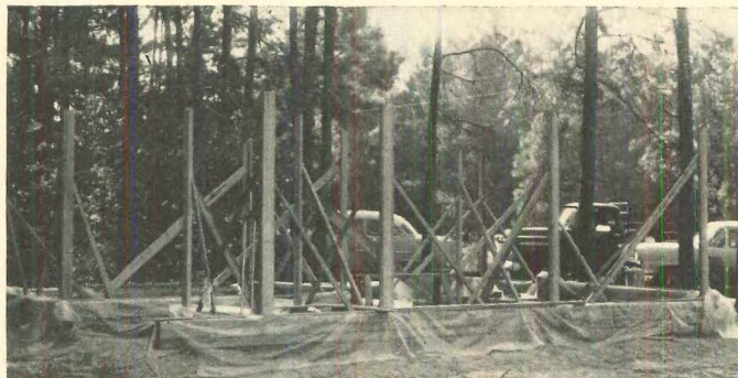
CORNER BRACES made of two 2x4's are set up to keep all walls in alignment until roof is placed. Polyethylene protects work from rain.
