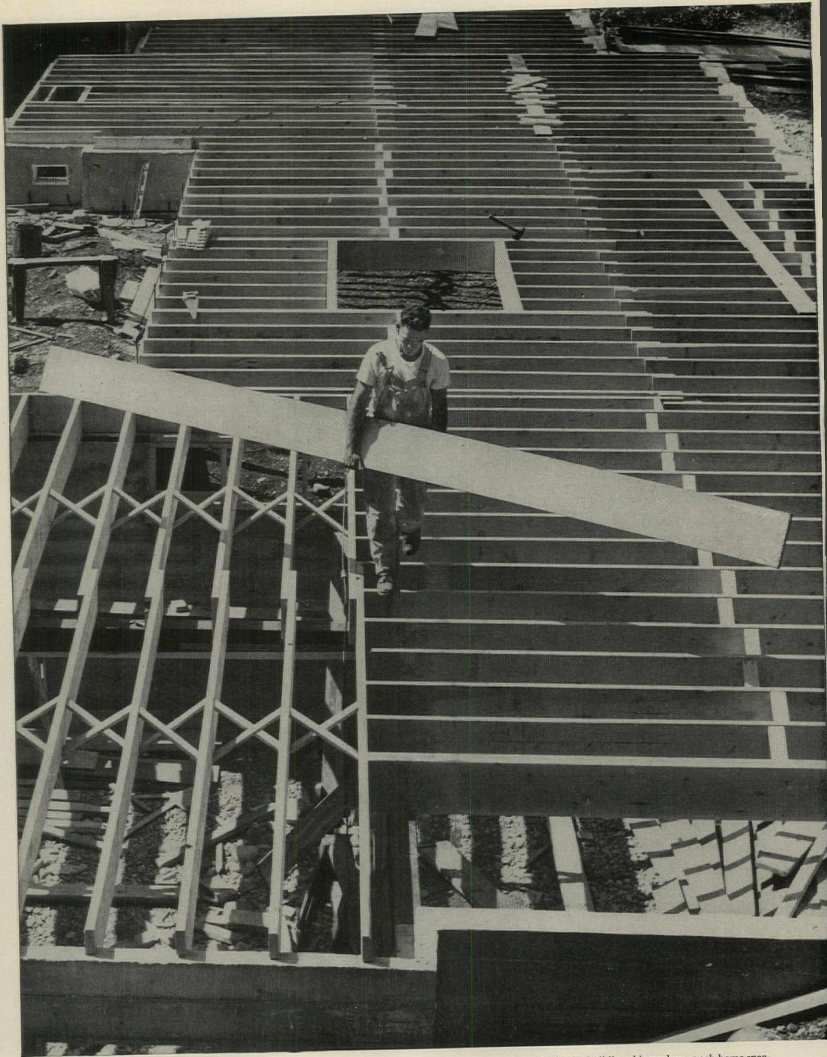
Like more and more homeowners, the family building this modern ranch home specified traditional joist construction with sub-flooring, to provide the comfort and beauty of hardwood floors. John Sutton, architect. Fister Construction, builder.
